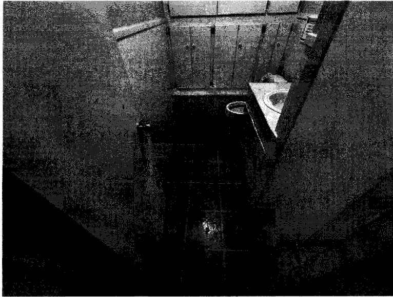
Photo 1 - Sheet Vinyl Flooring - Restroom
